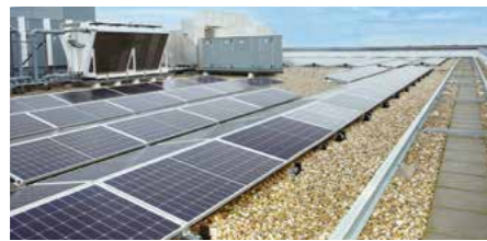
Rooftop solar panels installed by Vanderlande
