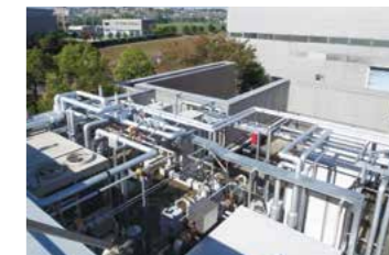
System using renewable thermal energy
